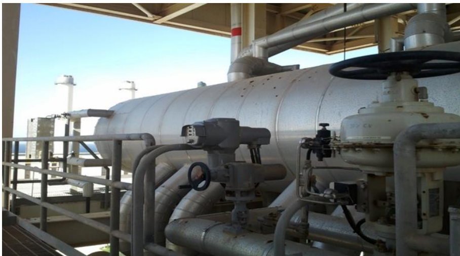
Figure 4. Low-pressure heat recovery steam generation tank in North Benghazi power station used high strength steel alloy ASTM A516-70
