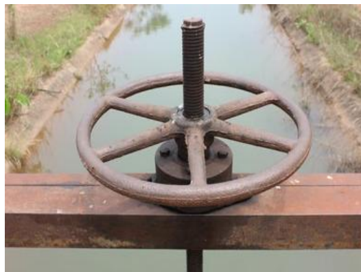
Figure 7. Sluice gate control wheel and jackscrew mechanism
