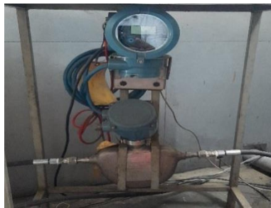
(c) Flow meter
