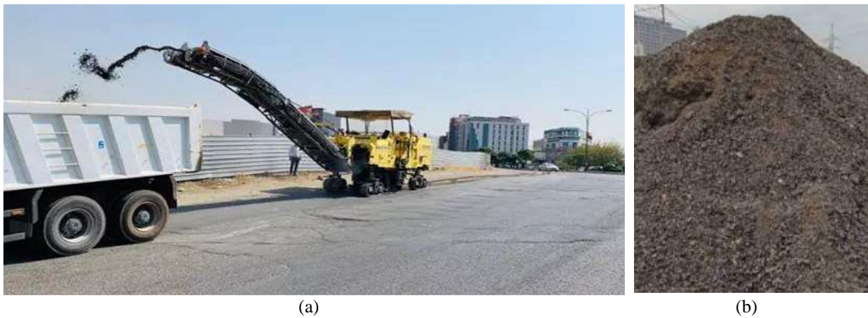
Figure 3. Source of recycled asphalt pavement aggregate (a) milling process of pavement, and (b) RAP stockpile)
