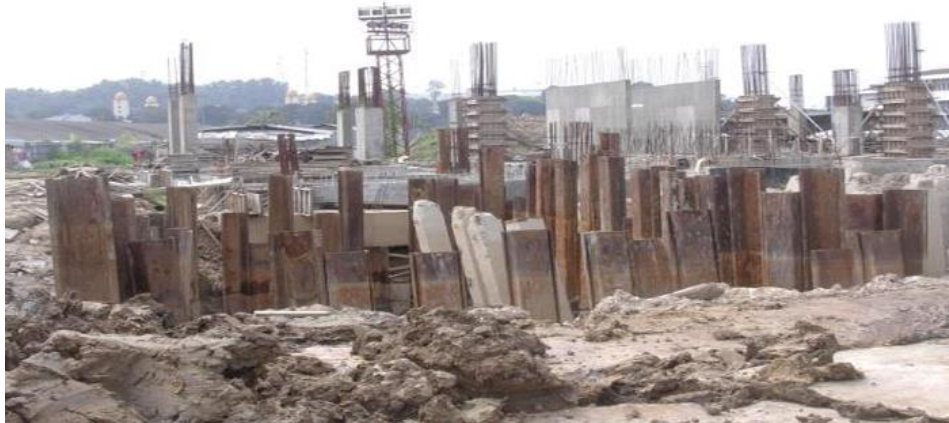
Figure 1. Sheet piles and piles adjacent to the excavation pit tilted
