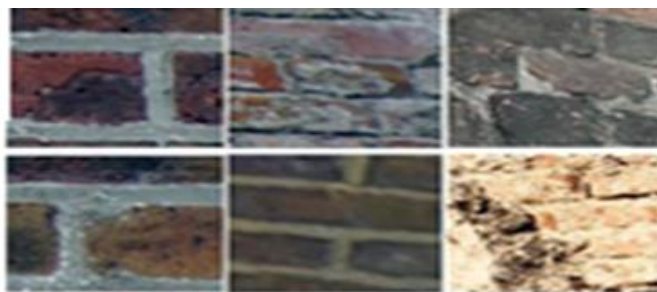
Figure 10. An example of non-crack patches.
