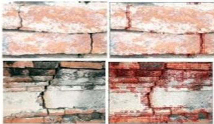
Figure 12. Crack localization of sample images.
