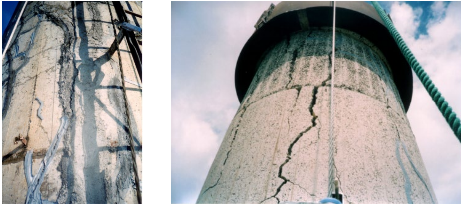
Figure 1. View of cracked chimney [4].
