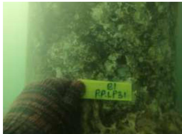
Figure 7. Presence of barnacles at submerged section
