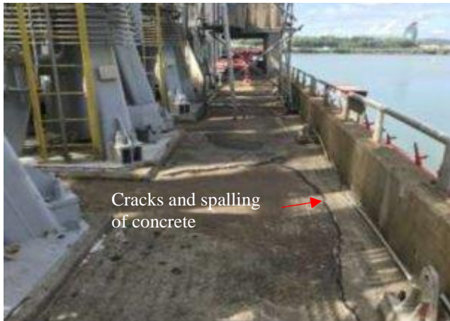
Figure 8. Minor cracks and spalling of concrete on loading platform
