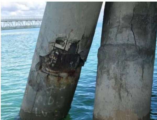
Figure 6. Major crack and spalling of concrete jacket due to chloride attack of steel reinforcement
