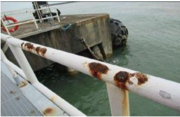
Figure 10. Surface corrosion on handrail
