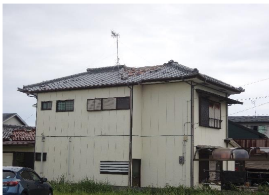
Figure 1. Damage to clay roof tiles (1).
