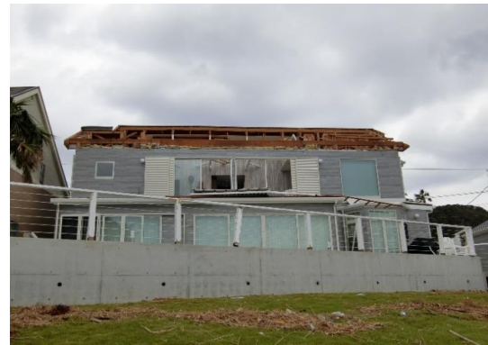
Figure 4. Damage to timber roof components (2).
