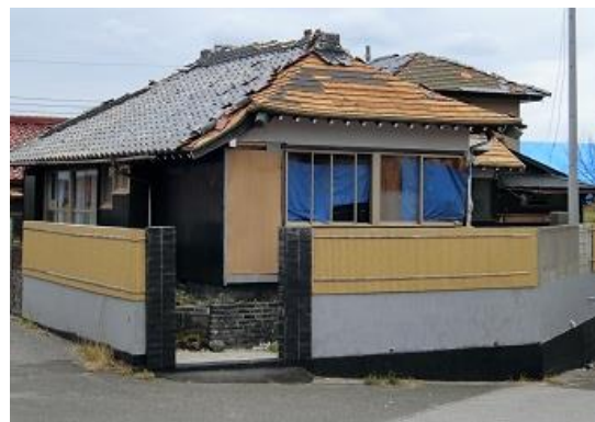
Figure 2. Damage to clay roof tiles (2).
