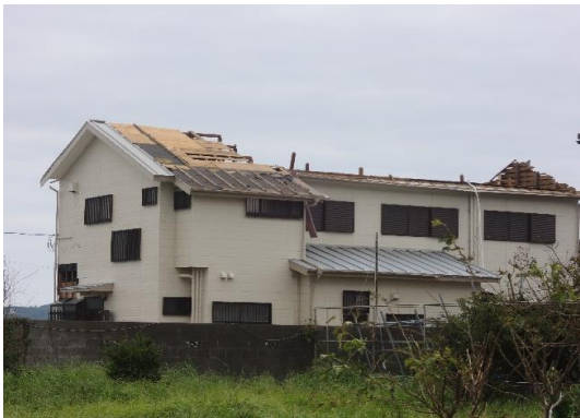
Figure 3. Damage to timber roof components (1).
