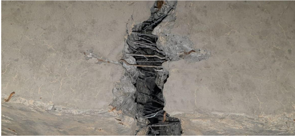
Figure 8. CMOD crack of the beam specimen with 40 kg/m 3
