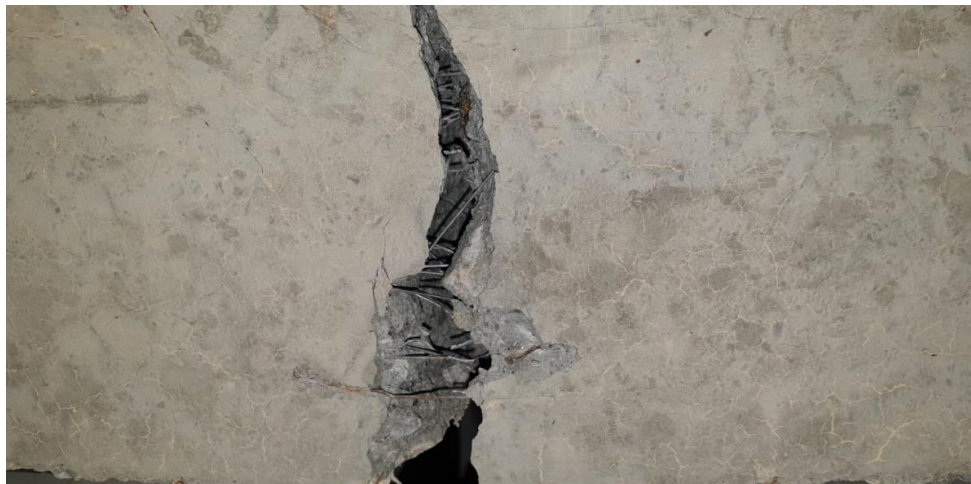
Figure 6. CMOD crack of the beam specimen with 20 kg/m 3
