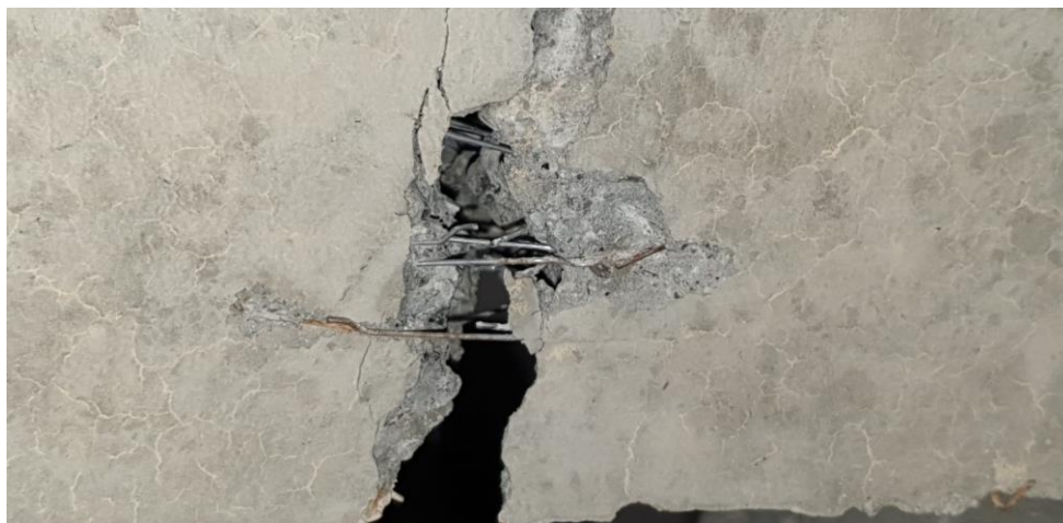
Figure 7. CMOD crack of the beam specimen with 30 kg/m 3
